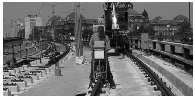
Figure 3: SFT inspector Mayk Hofmann at work during SFT inspections of track renewal in Dresden, Germany.
