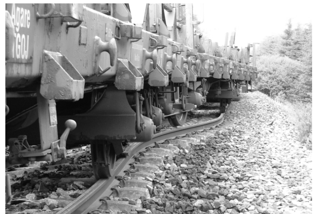
Figure 1: Picture of a transverse rail buckle due to inadmissible high longitudinal compressive load stresses.
